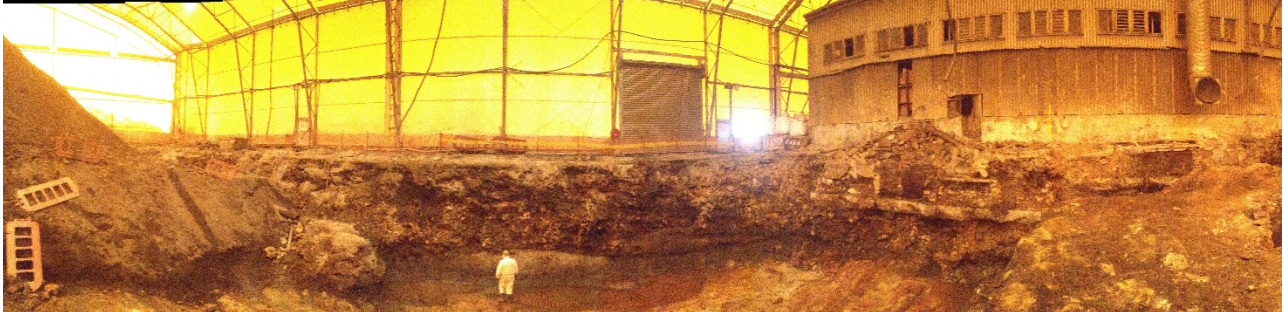
Figure 17: Panorama during excavation – centre facing the rear of the seawall (approx. 7m excavation depth and up to 6m below sea level), to the right is the underpinned Building No. 11.
