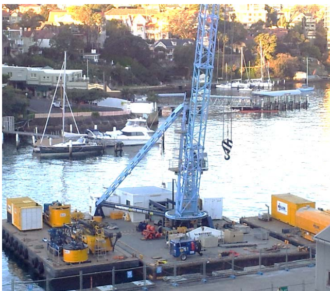
Figure 9: Most KGE plant and equipment was transported to/from site by barge and craned onto/off the wharf.
