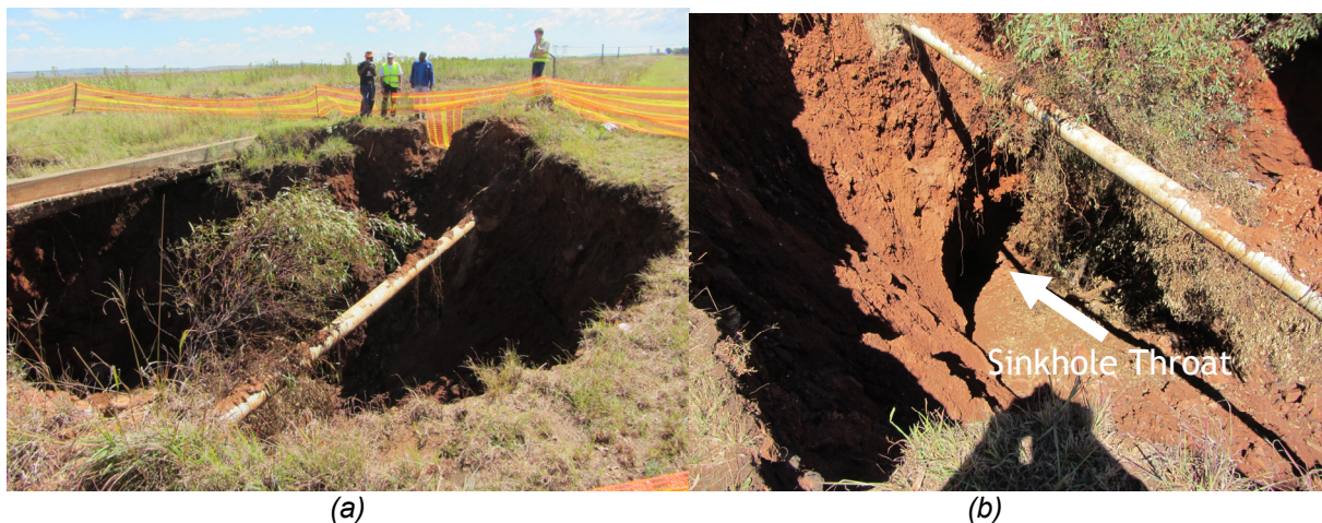
Figure 2. (a) Sinkhole; and (b) 1.5m Sinkhole Throat
